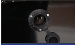
110-VOLT BATTERY CHARGER
